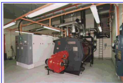
St Andrews CHP plant
